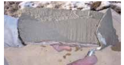
"Back-butter" the back of the stone with mortar before attaching to the scratch coat.
